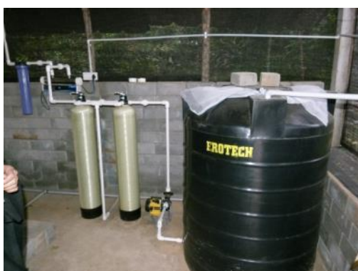
Water purification unit installed at certified estate
