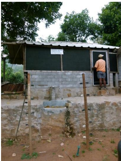
New water purification unit at certified estate
